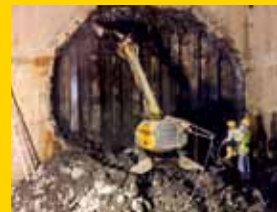
A six-meter hole through a reinforced concrete wall that's one and a half meters thick.
